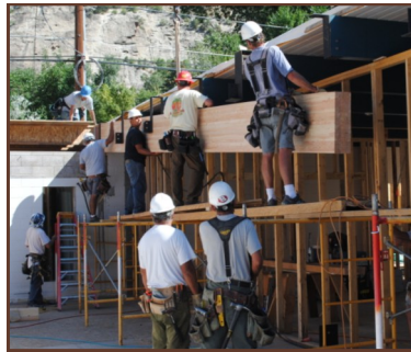
Workers put a new beam into place at the New Castle Branch Library.
