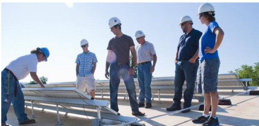
CMC students, along with Master Electrician Jordan Arnhold, watch as instructor Chris Ellis tests solar panels for an inspector.
