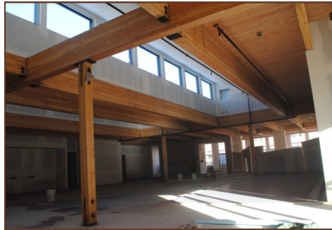
A sneak peek inside the New Castle remodel in mid December reveals natural light and beautiful beams.
