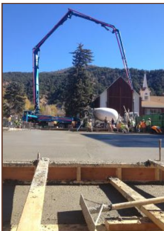
Photo taken during the 12 hour long post tension concrete slab pour in Glenwood Springs. You can view a time lapse video of the pour on our website.
